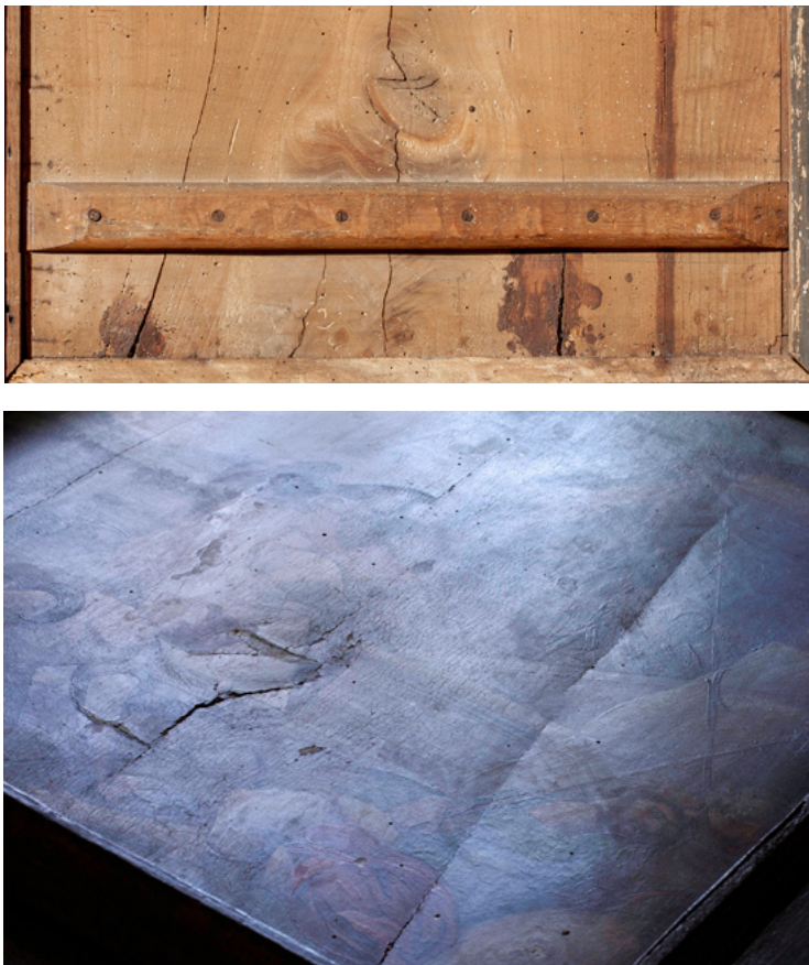
Figure 37. Fissures caused by the reinforcement of a panel, seen from the front and reverse. Photographs: IPCE Archive.
