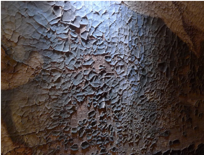
Figure 50. Flaking and lifting of the primer and pictorial layer. Photograph: Cristina Salas.
